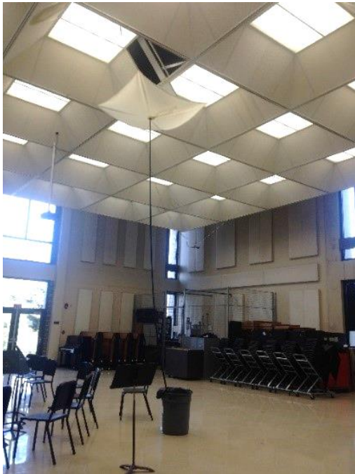
Ceiling leak (with improvised drainage system)
