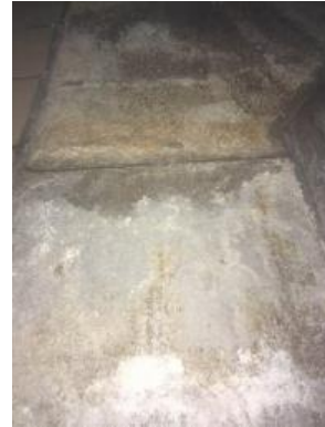
Water damage & efflorescence on limestone
