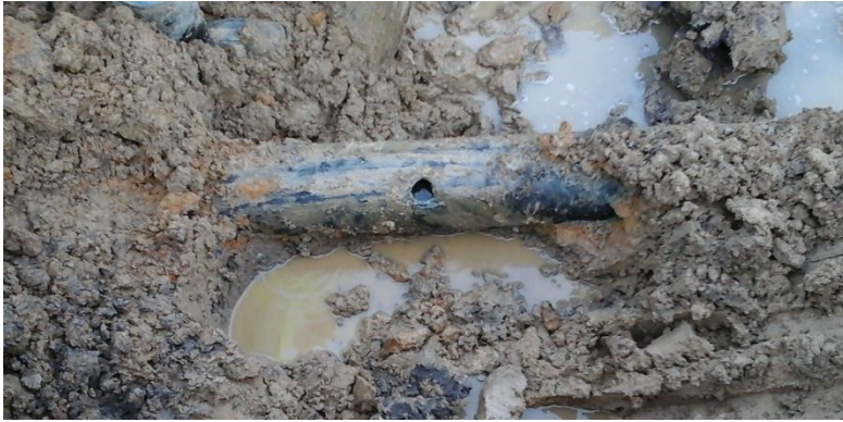
Water main break
